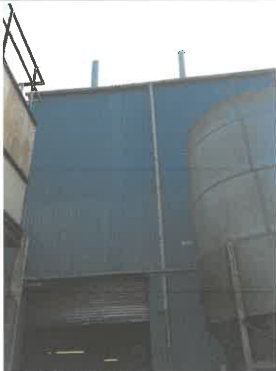
PHOTOGRAPH 2: S2 Cooler Plant Stack
