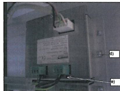
Figure 15 Installed ISB with its housing.
